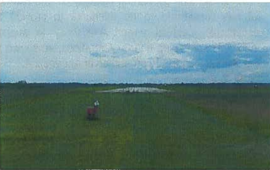
Simple Approach Lighting Fixtures (ODALS) fixtures and PAPI fixtures will require relocation to accommodate the extension of Runway 04-22 at both ends.
