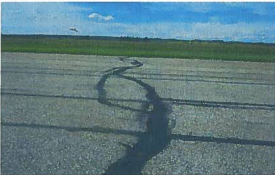
Longitudinal and transverse cracking on Runway 04-22.
