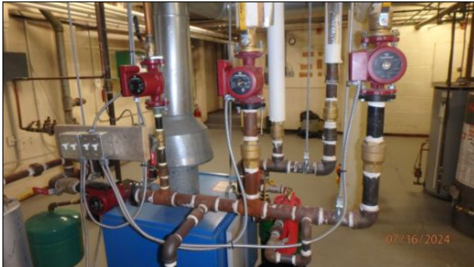
Boiler circulating pumps in good condition at time of inspection
