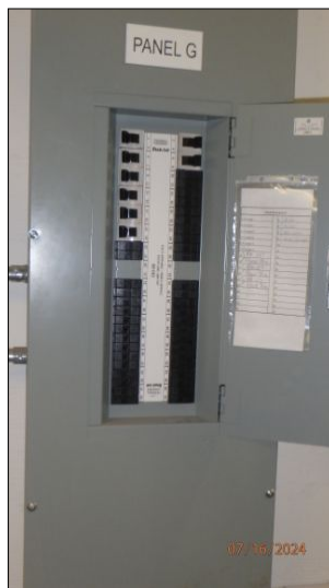
The building is equipped with 10 sub panels in various location. All visible subpanel exterior in good condition at time of inspection
