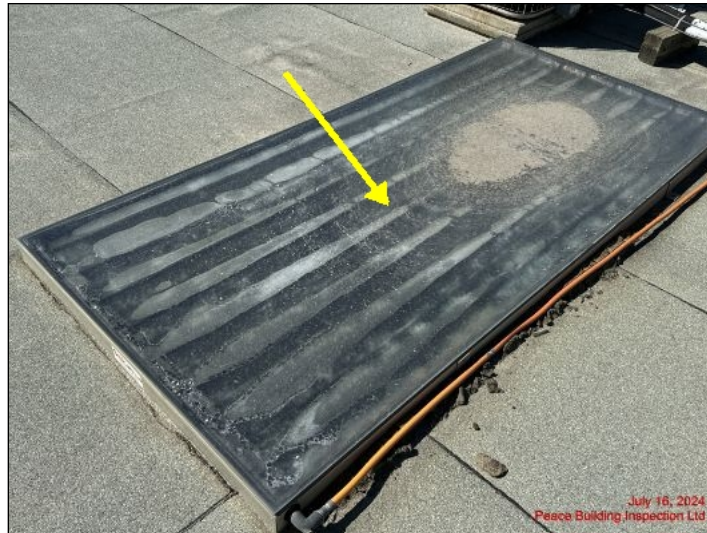
Solar water heater panel has failed. This solar panel will require replacement
