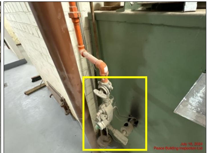
Gas line to wood stove needs to be removed and capped off
