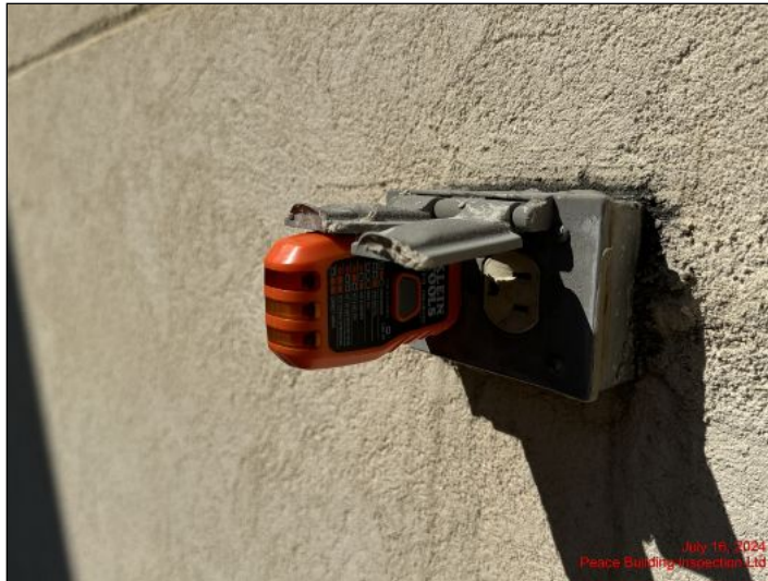
Exterior outlets did not have power when tested
