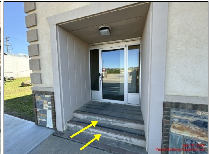
Some minor stair maintenance recommended at front of building
