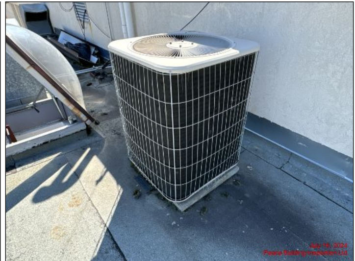
One air conditioner was not operational at time of inspection
