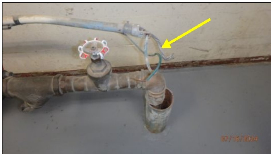
Main electrical service is not properly grounded at water line
