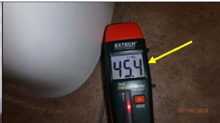
Some toilets were loose at floor and show signs of moisture
