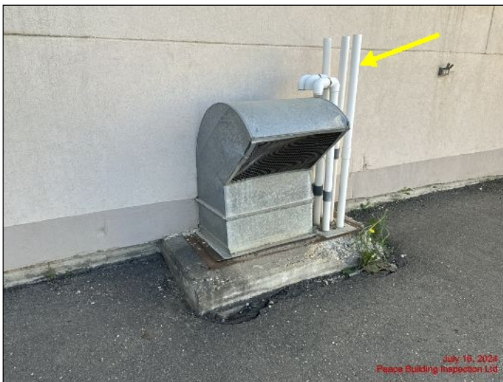
Furnace exhaust venting in good condition at time of inspection
