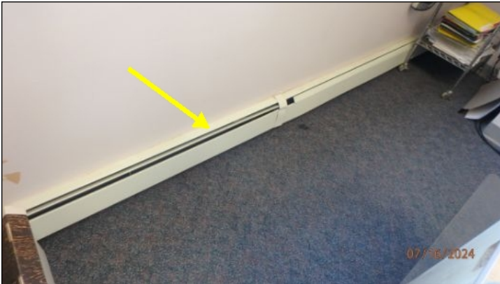
Building equipped with baseboard heaters
