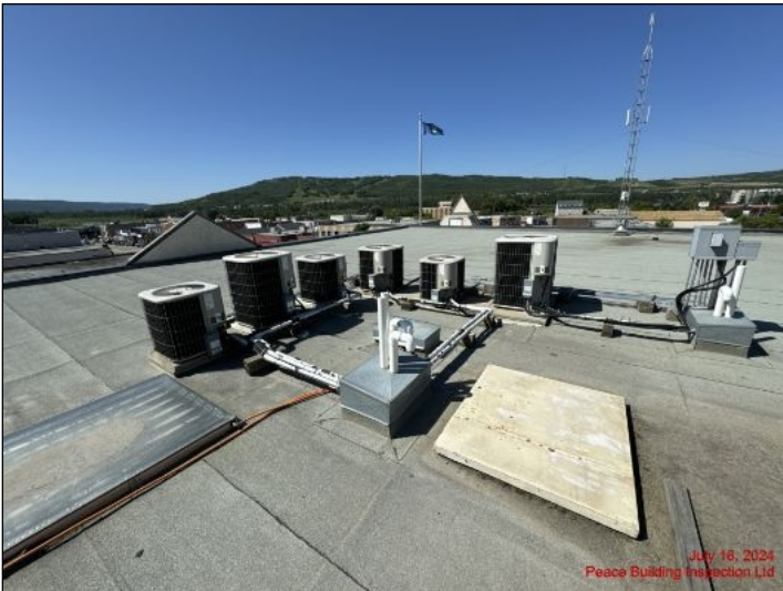
The building is equipped with 7 air conditioning units that are now 20 years old
