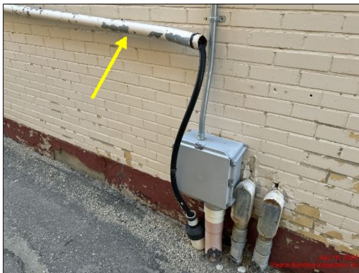
Exterior conduit requires proper attachment to building wall
