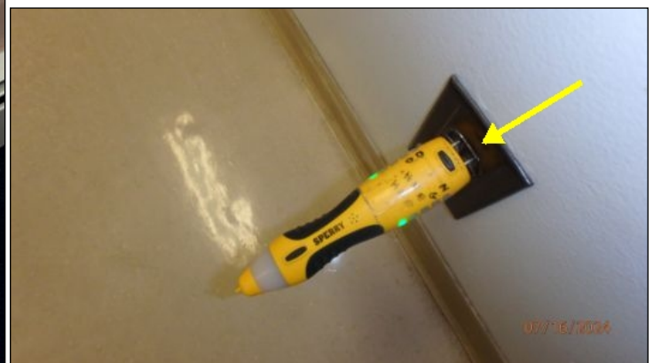
Several outlets are loose when a device is plugged in
