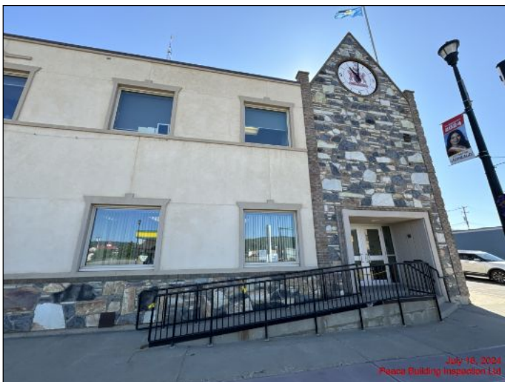
Front walkway ramp was sealed off at time of inspection
