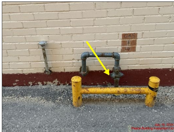
Gas line located at rear of building and properly protected from vehicle damage
