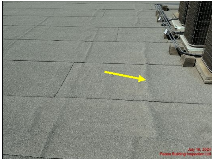
Ripples observed at roof in some areas. No roof leakage concerns visible at time of inspection
