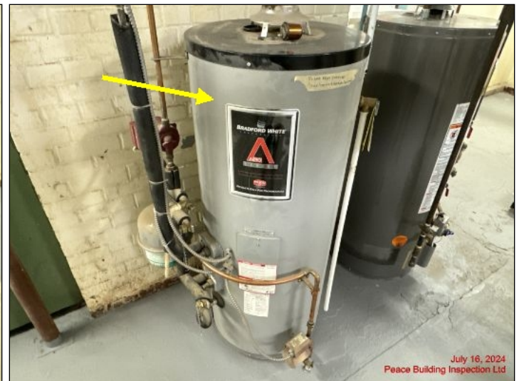
Solar water heater is not providing any heat input as the solar panel on the roof has failed
