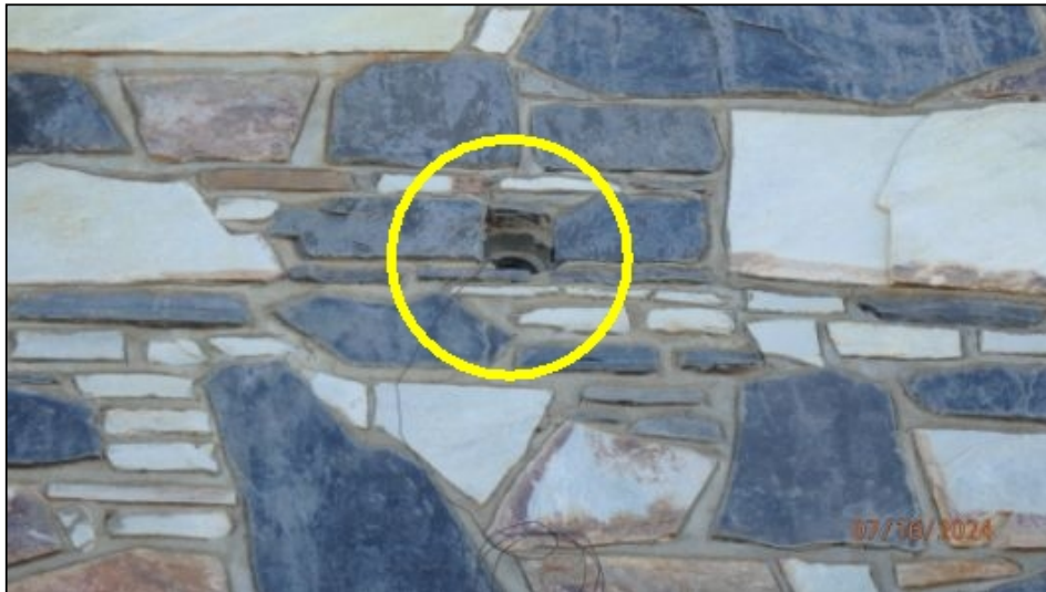
All exterior wall vents require screens to prevent bird entry
