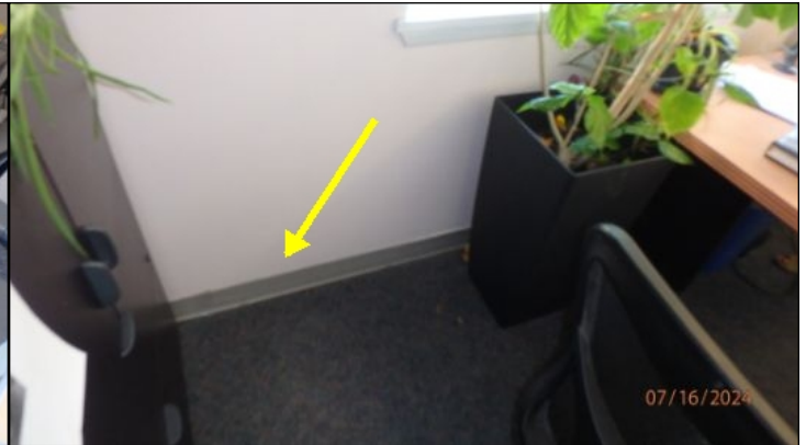
Some office areas are missing full wall baseboard heaters. Portable heaters observed in some office rooms for supplemental heat
