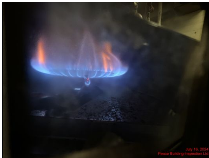
Water heater burner operated properly when tested
