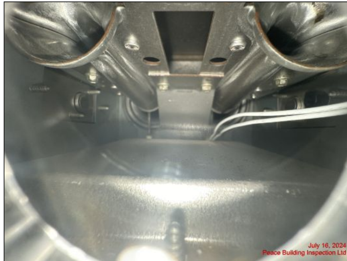
Visible portion of all furnaces in good condition at time of inspection
