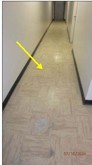
Some original floor tiles in basement may contain asbestos
