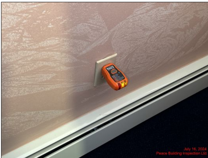
Board room area had several loose outlets
