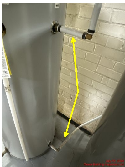
Solar water heater is provided with hot water from the conventional water heater
