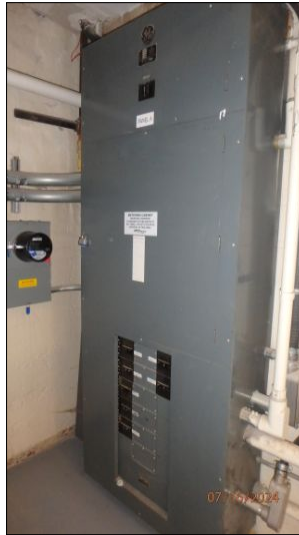
Building equipped with a 300 amp distribution breaker
