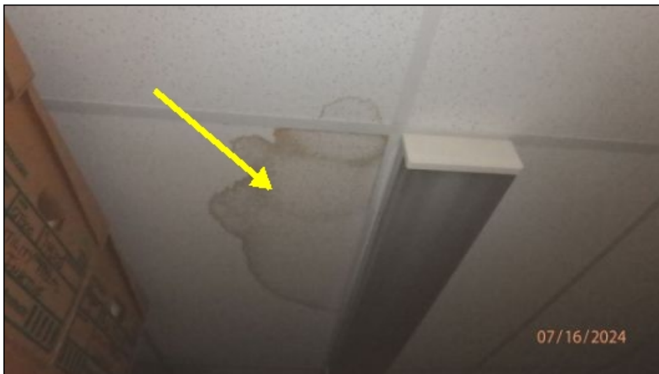
Basement ceiling storage area has some water stains
