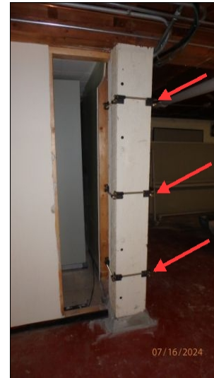
Wood support posts have engineered reinforcement that appear to perform as intended
