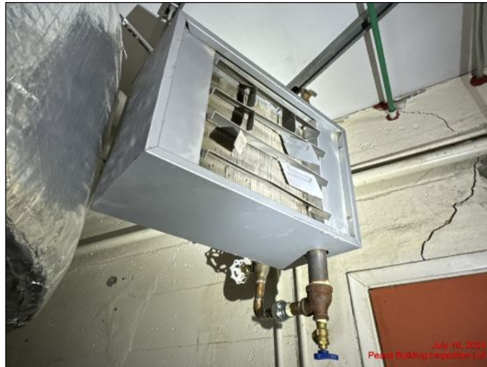
Basement equipped with hot water radiant overhead heaters in good condition at time of inspection
