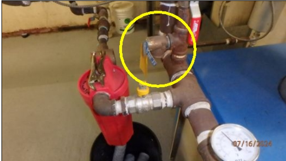
Boiler pressure relief valve should terminate at the floor level
