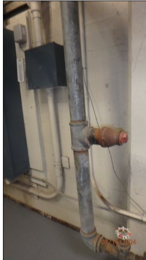
Some building water supply pipes are galvanized
