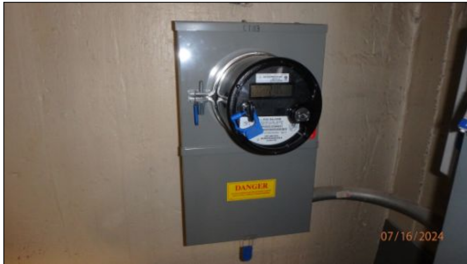
Electrical meter located in basement boiler room
