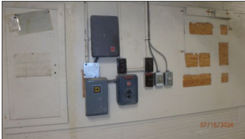
Boiler and system shutoff properly located
