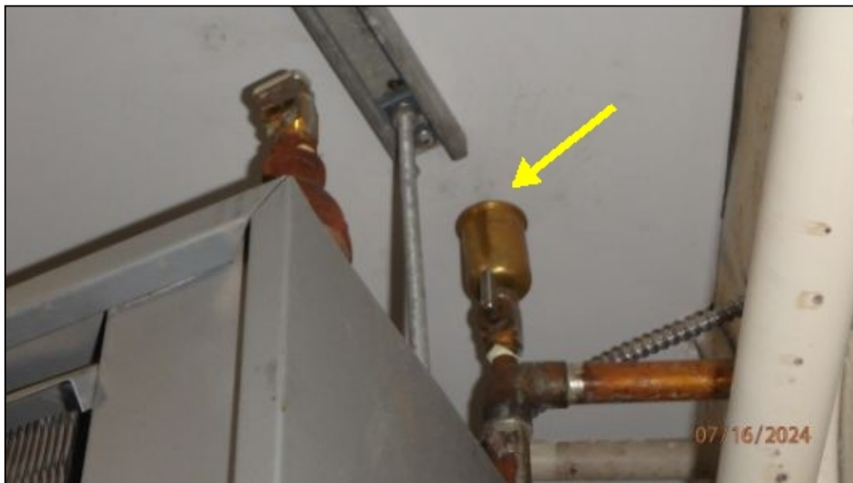
Visible boiler air vent in good condition at time of inspection
