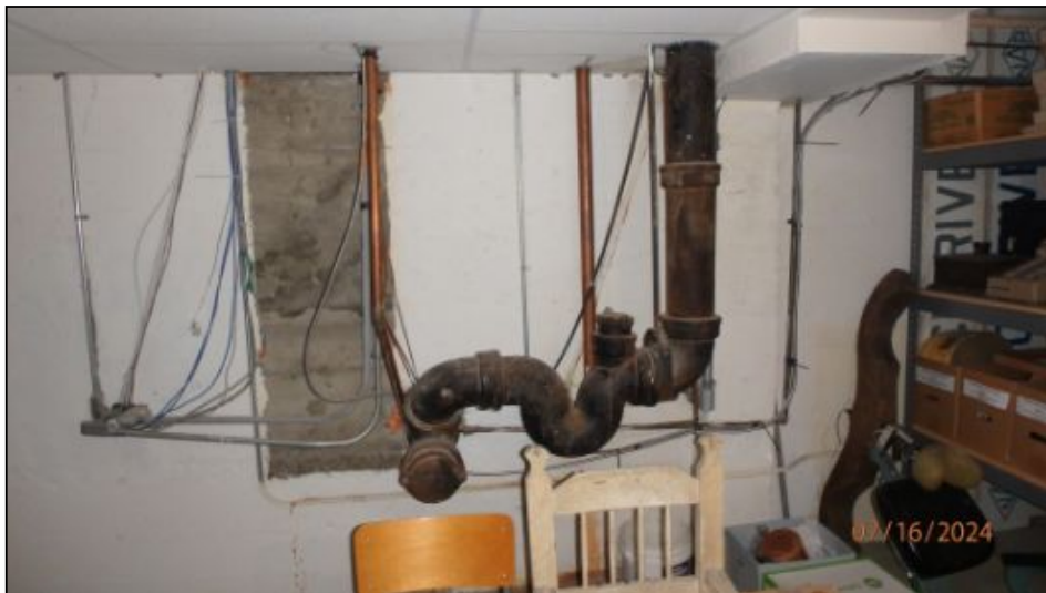
Building equipped with cast iron sewer piping. Normal life is 50 years
