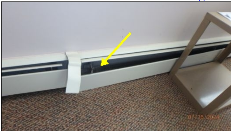
Several baseboard heater covers are loose or damaged
