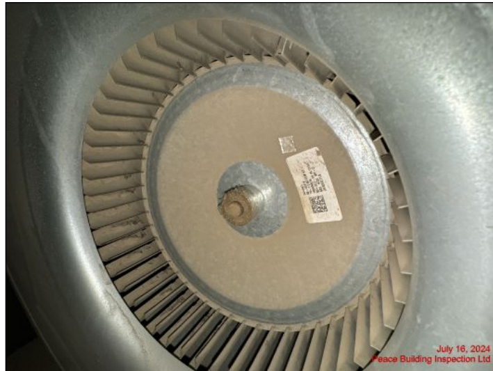
All furnace blowers and motors in good condition at time of inspection
