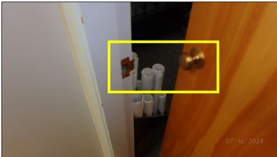
Several interior doors do not latch closed
