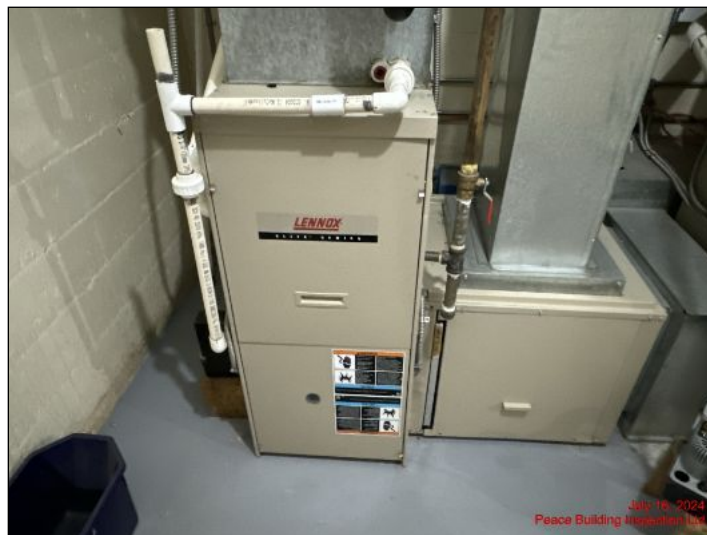
All furnaces in good condition at time of inspection
