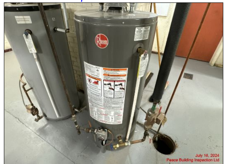
5 year old conventional water heater in good condition at time of inspection
