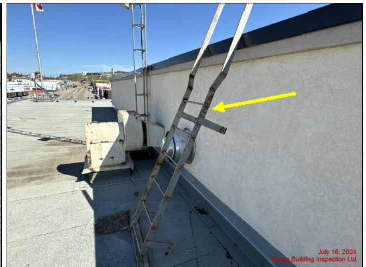
Roof access ladder is not properly installed. Adequate anchor to building is required for safety reasons
