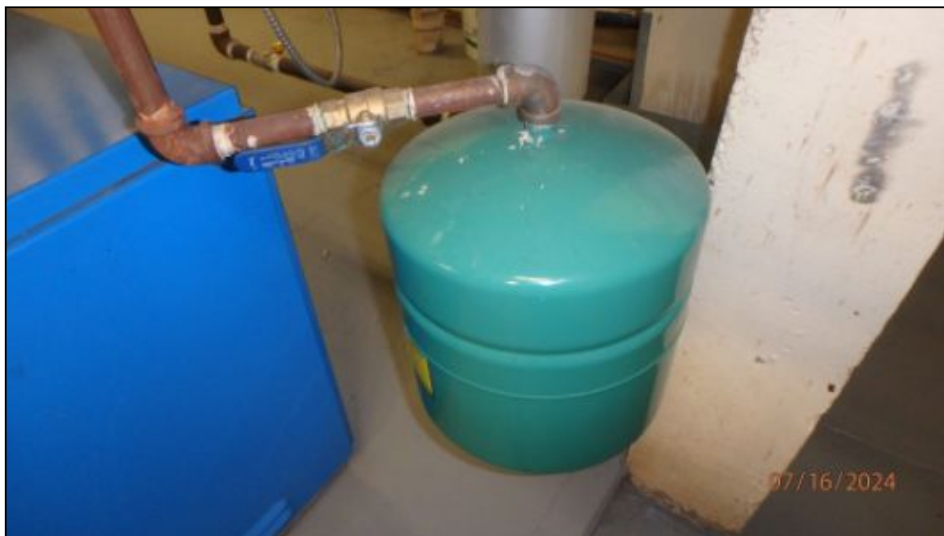
Boiler expansion tank in good condition at time of inspection
