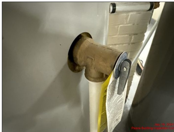
Water heater pressure relief valves in good condition at time of inspection
