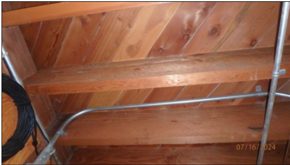
Wood boards over conventional joists in good condition at time of inspection
