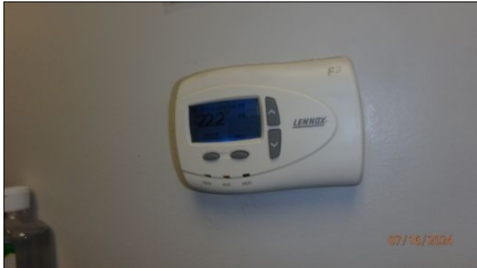
Some thermostats were not properly located
