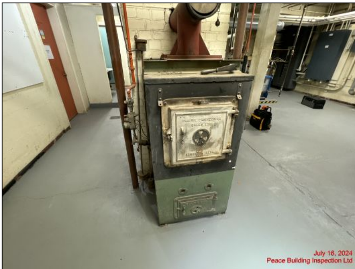
Building equipped with a wood stove that is no longer used and not fully inspected
