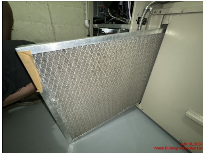
Furnace air filters in good condition at time of inspection
