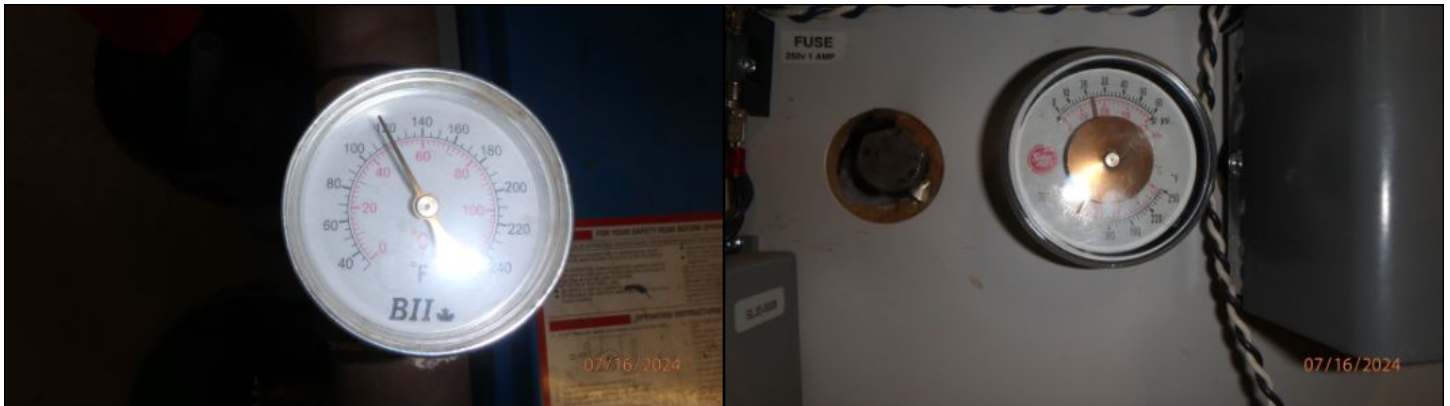
Boiler operating at proper temperature
