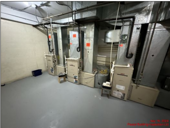
The building is equipped with (7) twenty year old furnaces
