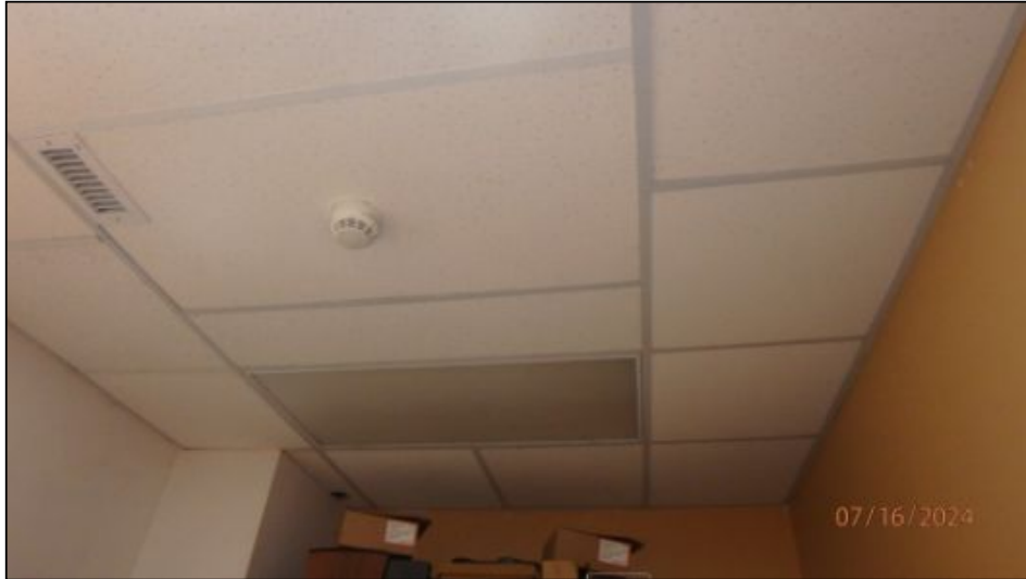
Ceiling tiles are not removed to avoid damage
