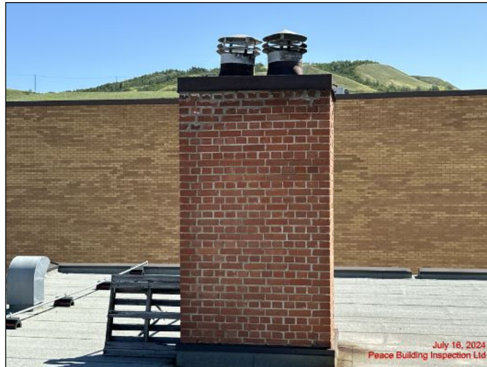
Boiler exhaust flue in good condition at time of inspection
