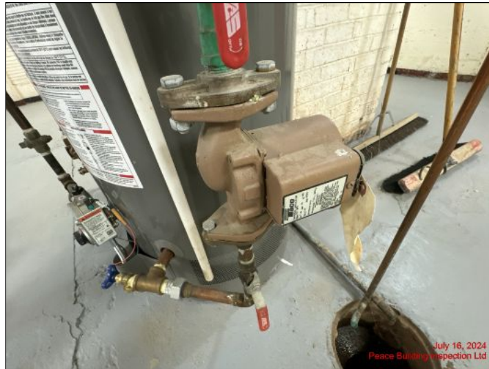
Water heater Circulation system operated properly at time of inspection
