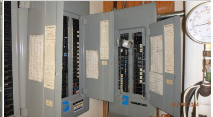
(3) Service panels located in upper level mechanical room
