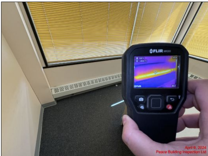
Most baseboard heaters were operational at time of inspection
