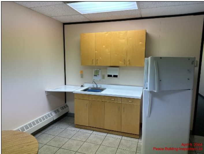
Lower level kitchen/Break Room sink requires repairs
