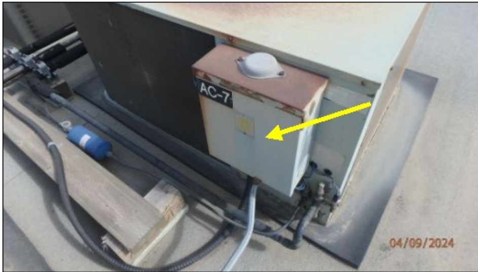
Each air conditioner equipped with a local disconnect as required
