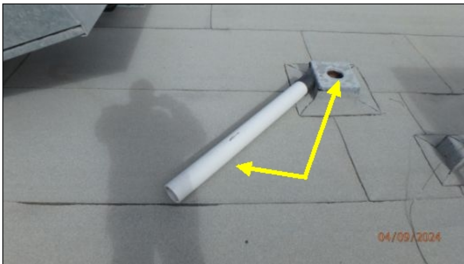
One plumbing vent stack needs to be attached
