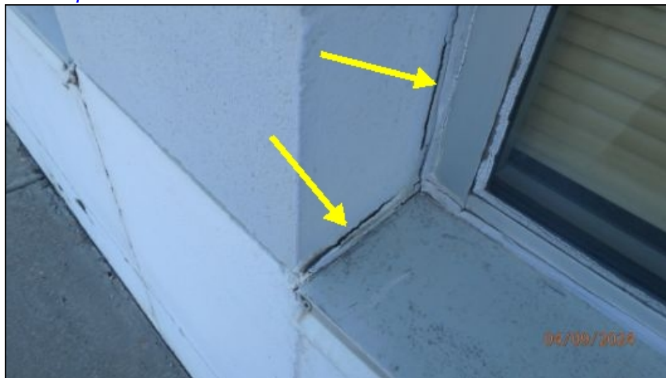
Exterior window trim requires improved sealant to prevent leakage
