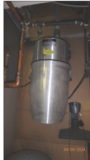
Central vacuum systems are not inspected
