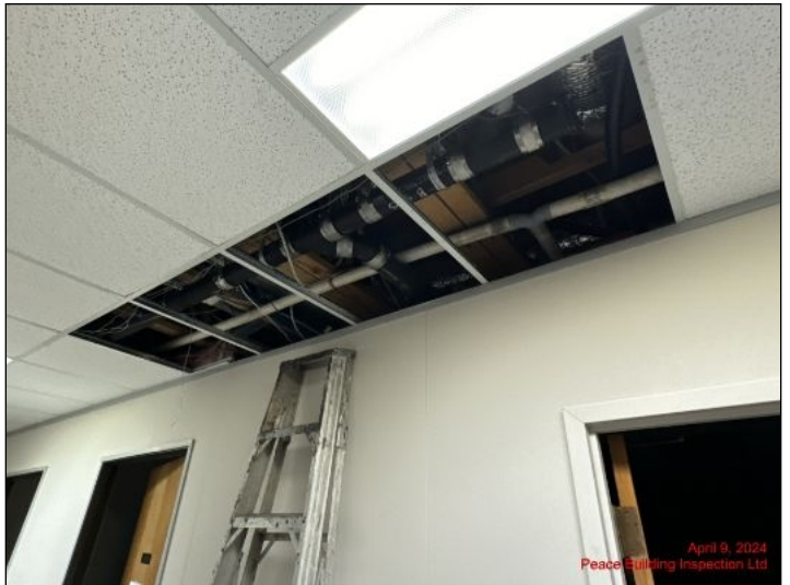
Damaged or missing ceiling tiles from past leakage repairs
