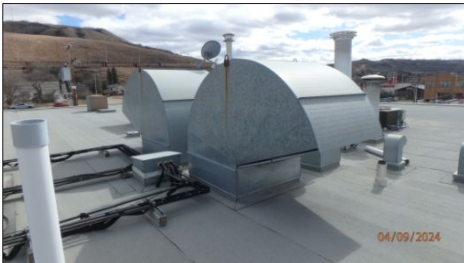
Fresh air intake in good condition at time of inspection
