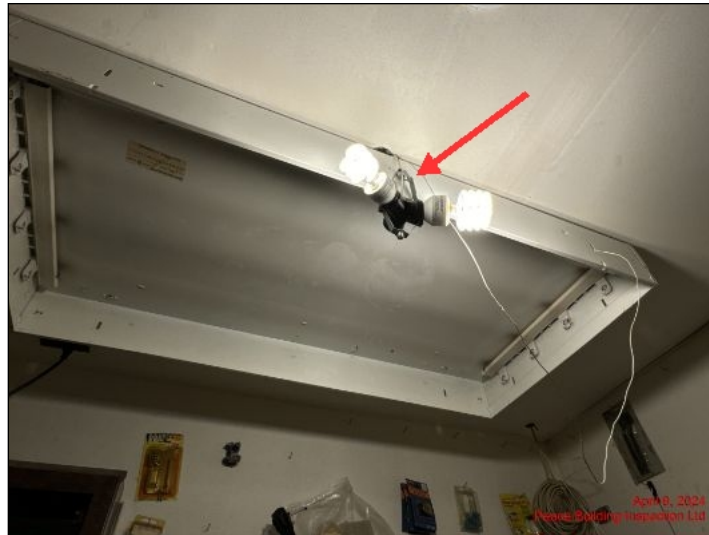
Poor light ballast installation observed at lower level maintenance shop
