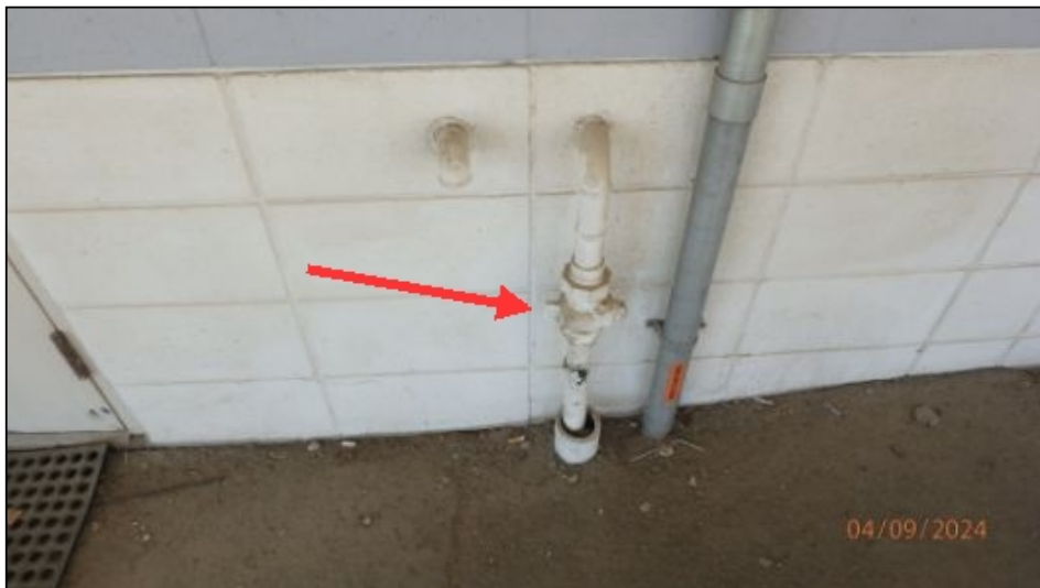
Main gas shutoff located at rear of building
