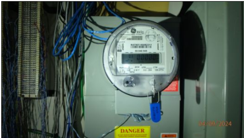
Electric meter located at rear electrical room. Meter in good condition at time of inspection
