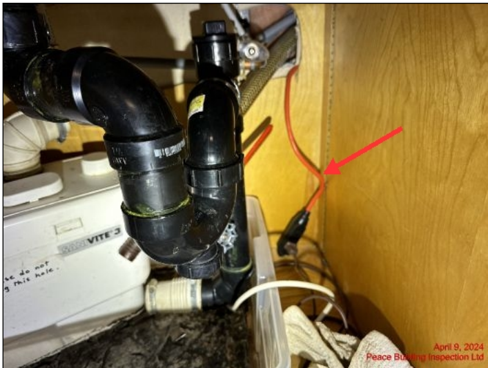
Extension cord used for permanent wiring under lower level kitchen sink drain lift pump
