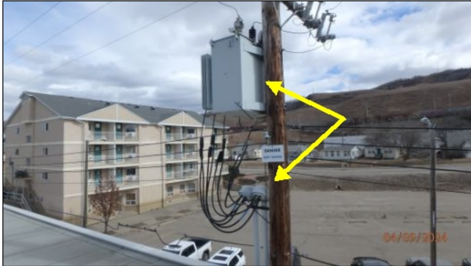
Overhead power supply in good condition at time of inspection
