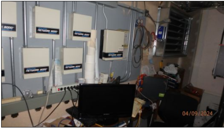
Low voltage systems are not inspected
