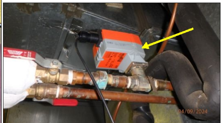
Some baseboard heaters had no heat at time of inspection. Some zone valves likely need replacement
