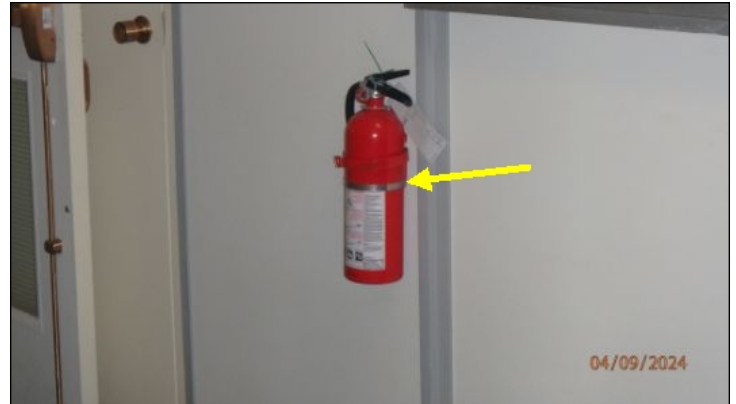
Fire extinguishers are not inspected
