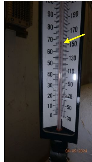
Boilers operating at proper system temperature
