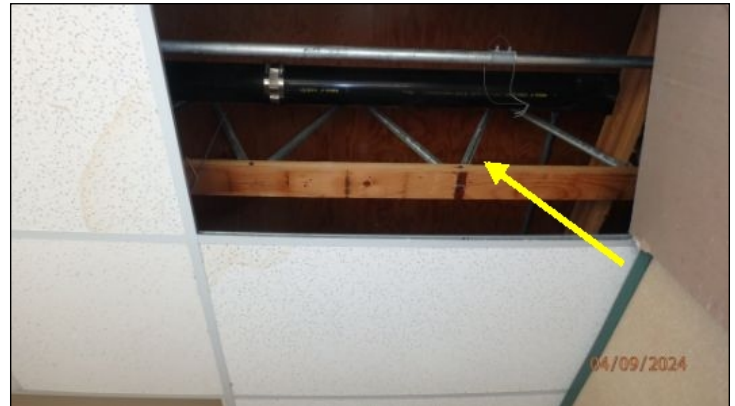
Roof truss joist structure support appears in good condition at time of inspection
