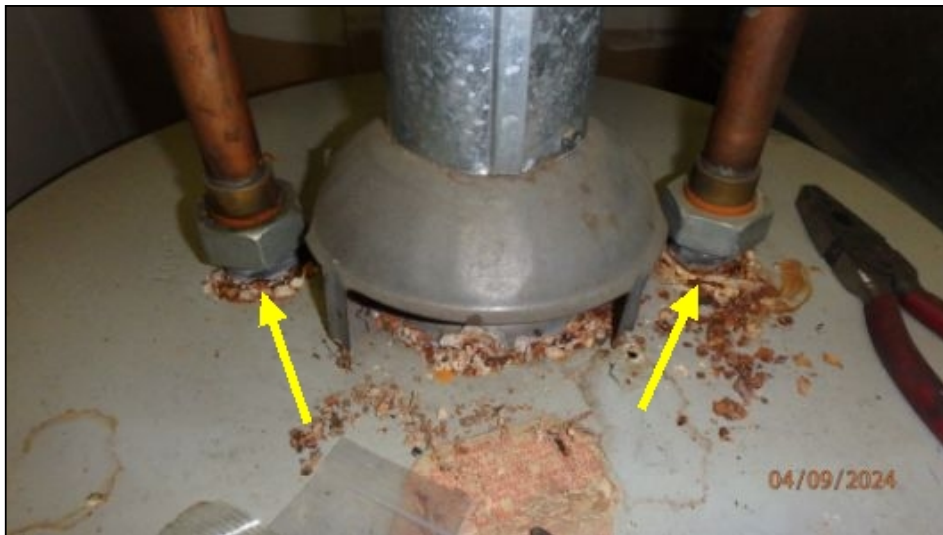
Water heater pipe connections are severely corroded. Tank replacement recommended
