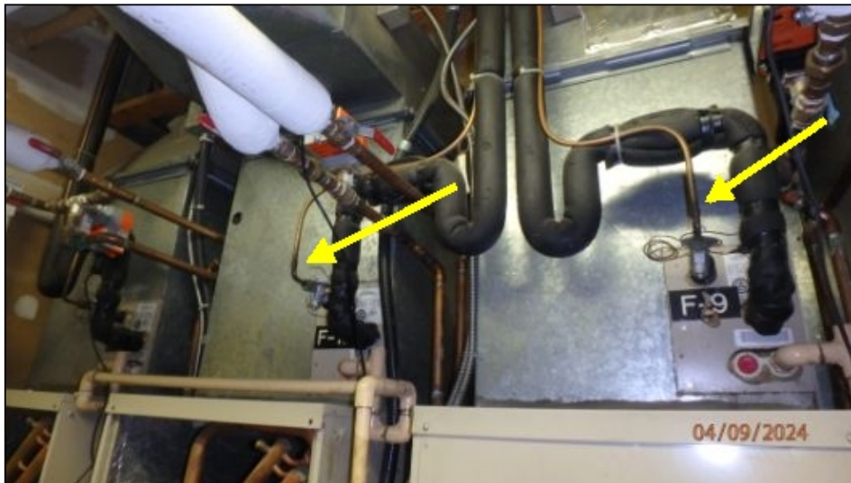
Air conditioner evaporator coils are not accessible for inspection
