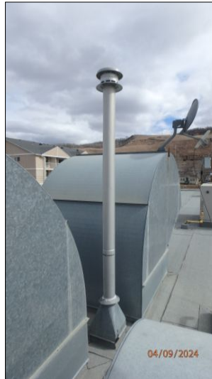
Water heater exhaust flue in good condition at time of inspection
