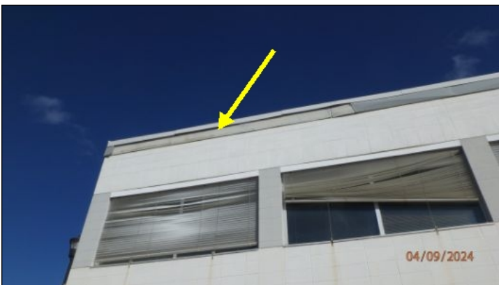
Southwest corner of building is missing a 10 foot section of fascia
