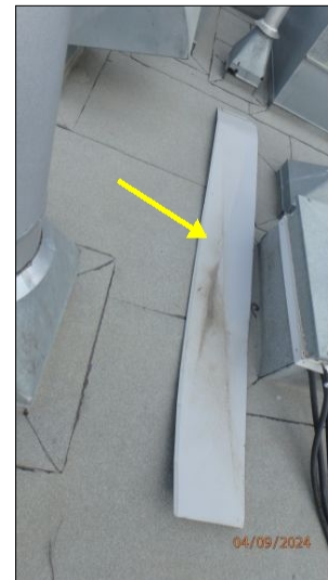
Missing fascia was located on roof of the building
