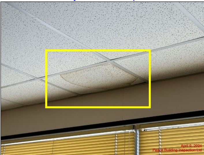
All lower level ceiling stains were dry at time of inspection
