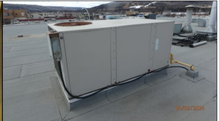
Building is equipped with an older HVAC unit. Unit label was missing. Inspector unable to determine age. Further investigation recommended for this unit
