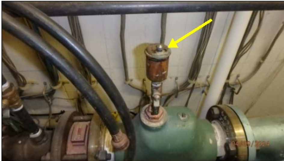
Boiler air vent in good condition at time of inspection
