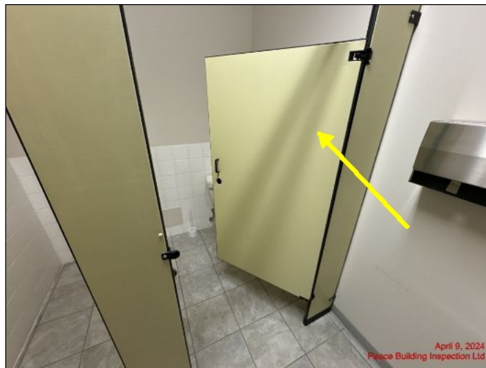
One lower level bathroom door is very loose at hinge
