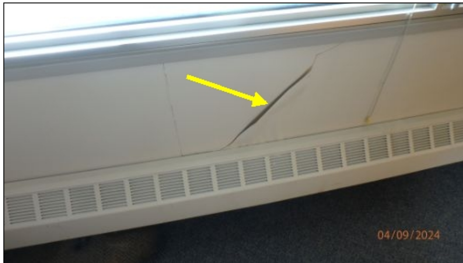
Room #245 has some minor wall damage that requires repair before painting
