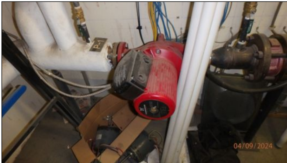
Boiler circulating pump in good condition at time of inspection
