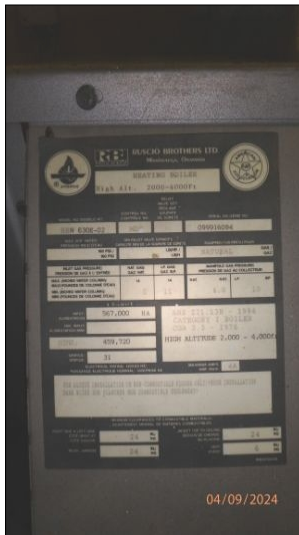
Boiler #1 Data Plate
