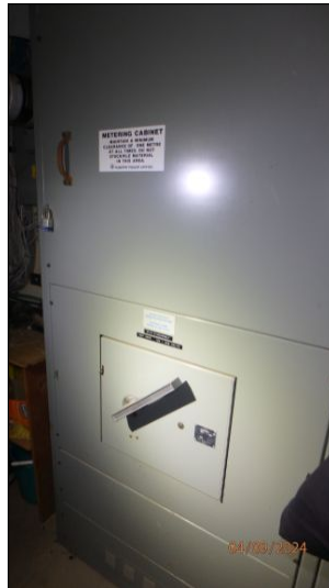
Building equipped with a 600 amp main breaker
