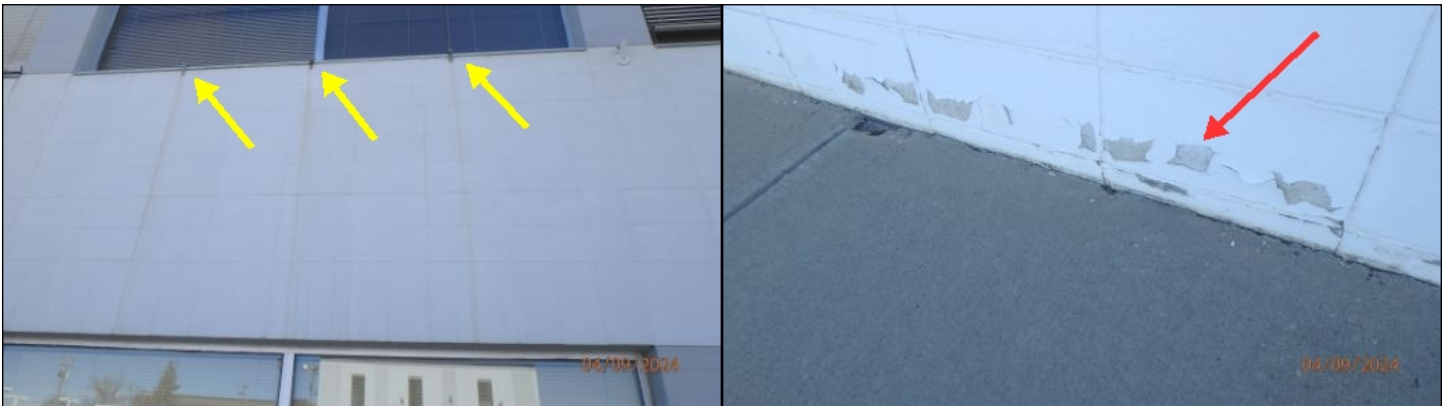
Exterior walls requires some scraping and painting to protect the concrete block walls
