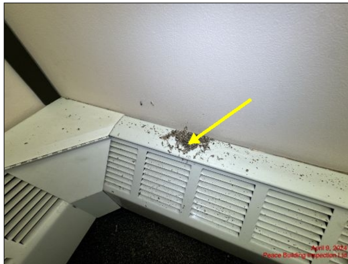
Concrete block walls are insulated with vermiculite which may contain asbestos
