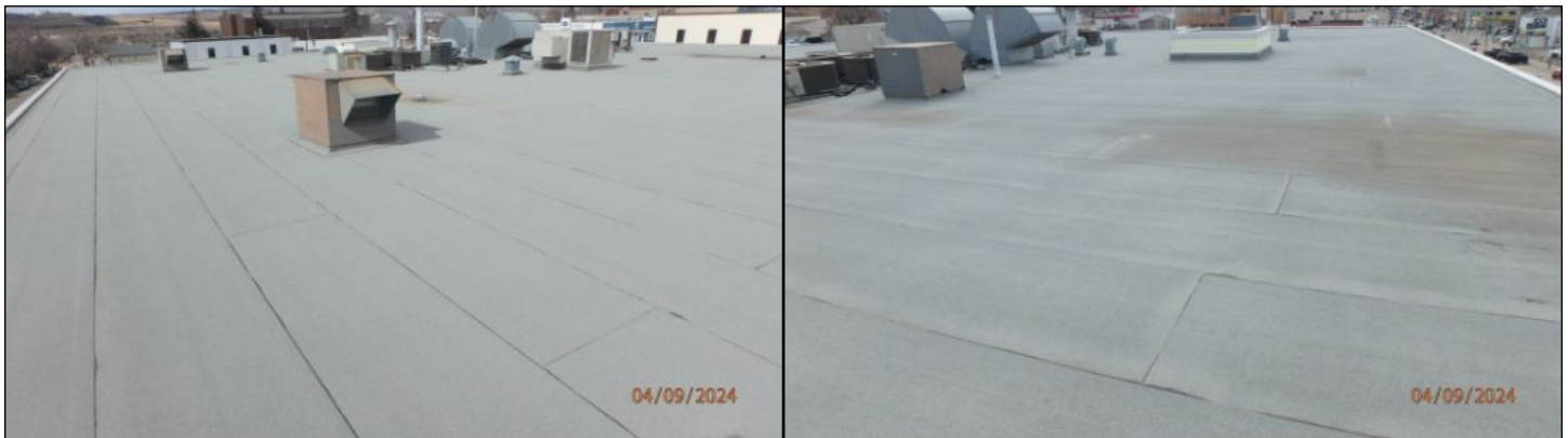
Roof cover in good condition at time of inspection Roof cover age was not determined but appears in good condition at time of inspection
