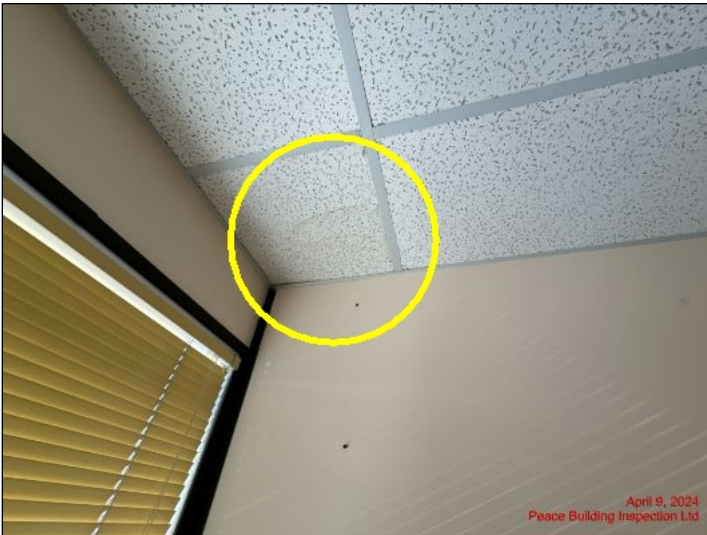
Some lower level ceilings show water stains that were dry at time of inspection
