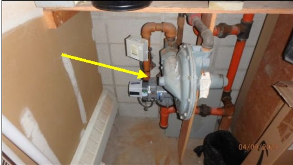
Gas meter located in rear electrical room
