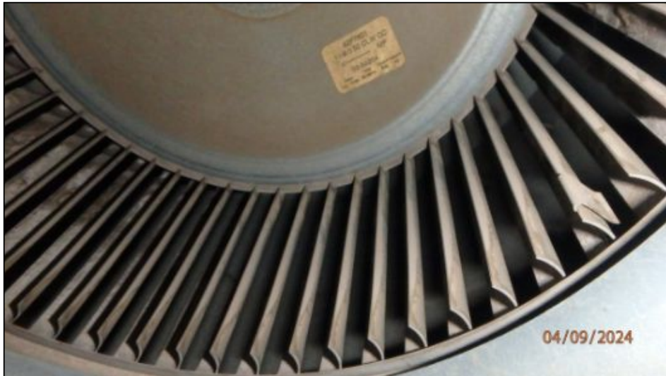
All furnace blowers appear in good condition at time of inspection
