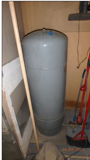
Boiler expansion tank in good condition at time of inspection
