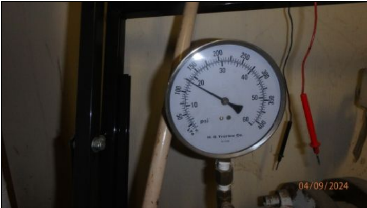
Boiler system operating at proper pressure at time of inspection
