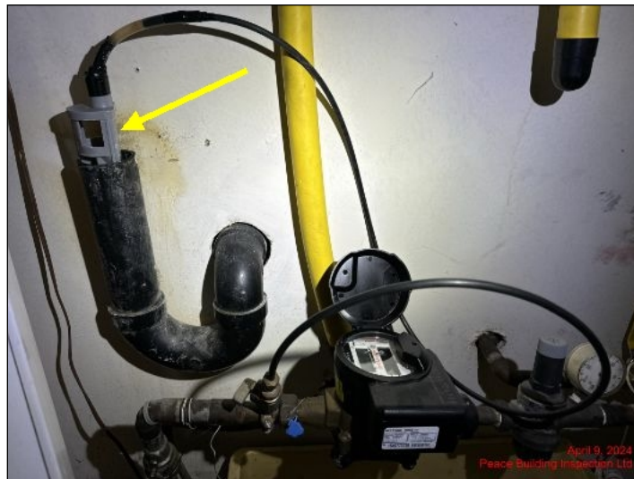
Building equipped with anti freeze water dribble line
