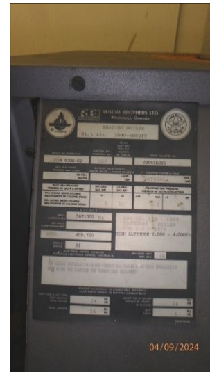
Boiler #2 Data Plate
