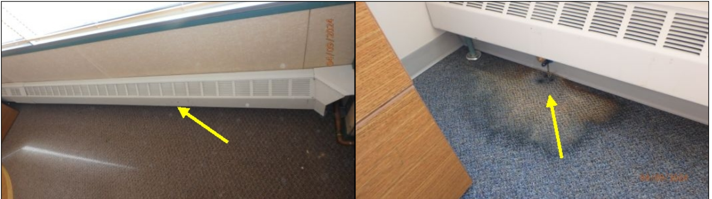
Several radiant baseboard heaters did not provide heat. Further investigation recommended
