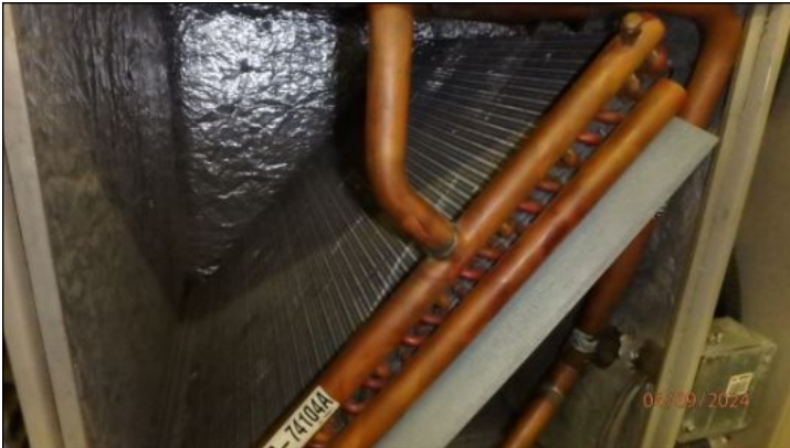
No visible concerns observed at the furnace radiant heaters
