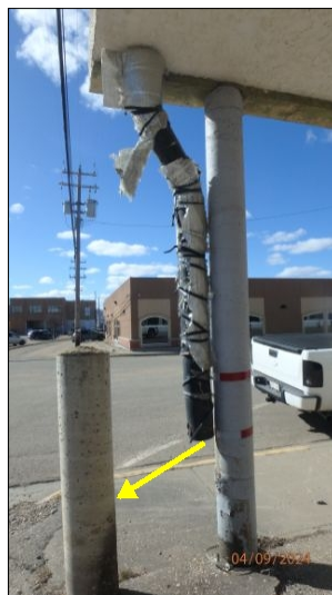
Rear downspout should drain away from the structure support post
