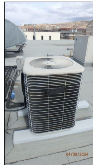
Building has (3) newer air conditioners that appear in good condition at time of inspection
