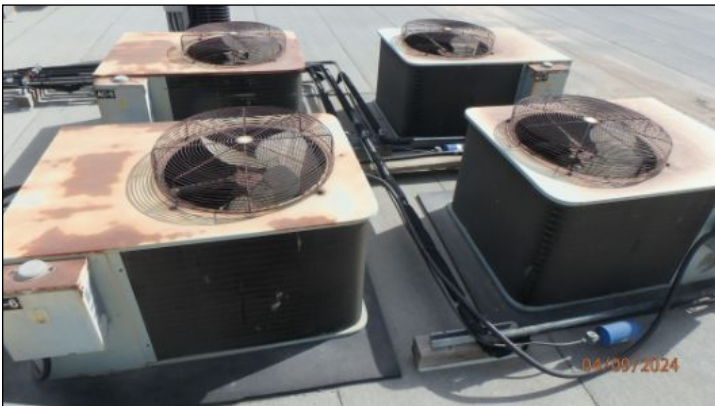
Building equipped with (11) air conditioning units. (8) of the units are at or very near the end of service life. Replacement likely needed
