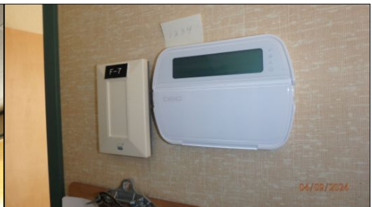
Alarm systems are not inspected
