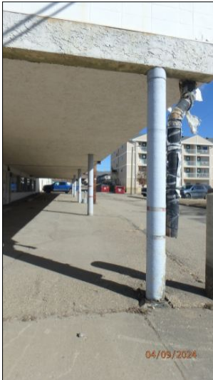
Rear parking lot overhang support in good condition at time of inspection
