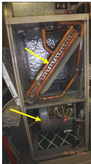
Boilers provide heat to each furnace radiator that in turn has a blower providing heat to each building zone
