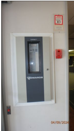
Alarm systems are not inspected
