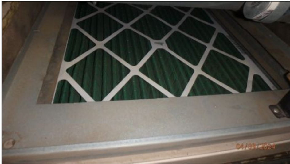
Each furnace air filter should be replaced every 3 months
