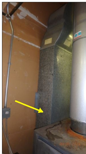
Mechanical room properly equipped with combustion air
