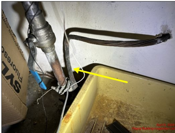
Electrical service is grounded to the water supply inlet
