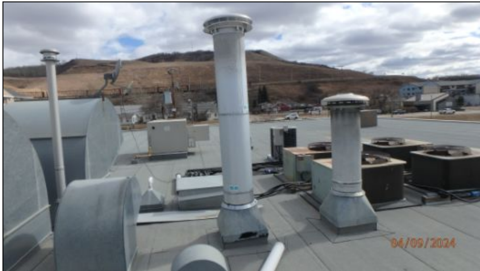
Boiler exhaust flue in good condition at time of inspection
