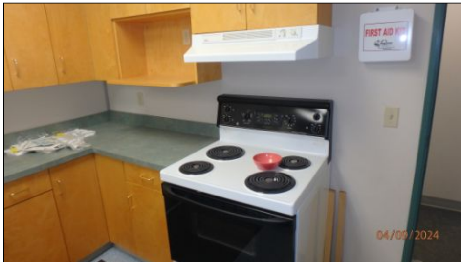
Upper level kitchen stove exhaust vent in good condition at time of inspection
